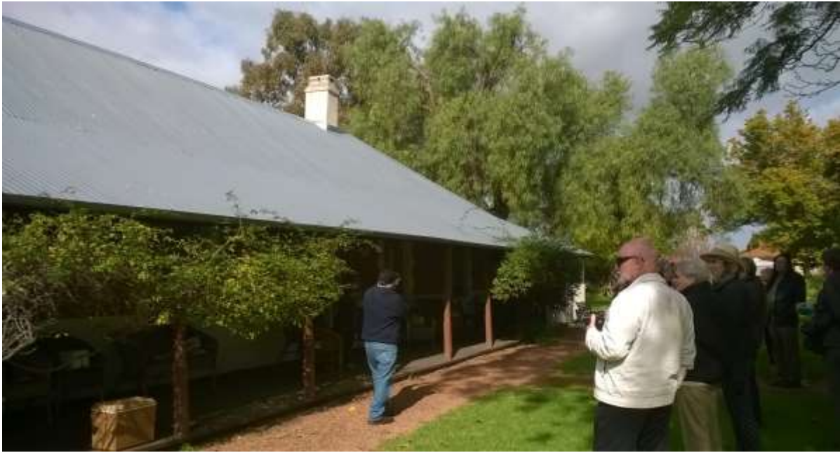
A sound roof is the best protection for heritage buildings. Old Blythewood also has the benefit of an attentive Resident Warden in Vince Taylor.
